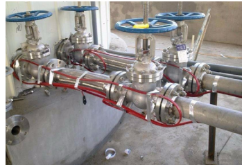
Pipe Heat Tracing
